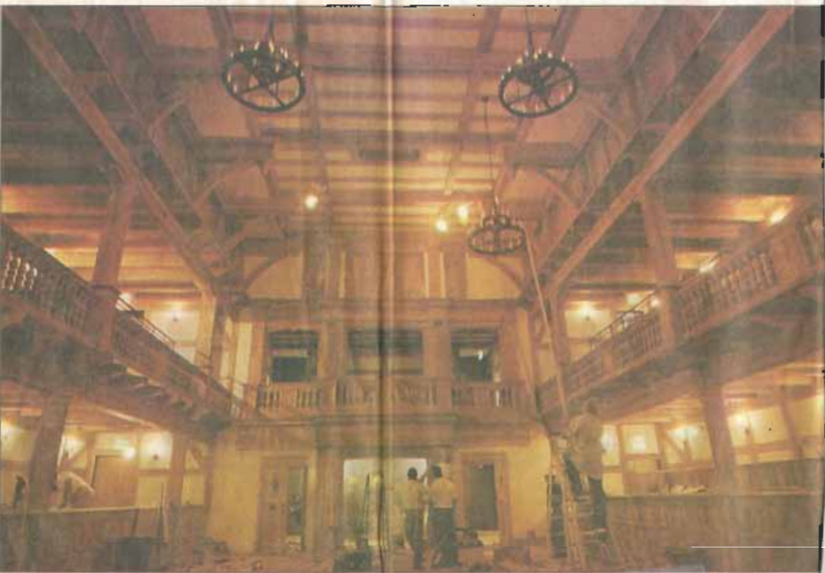
A workman (right) steadies a chandelier being raised at Blackfriars Playhouse. The playhouse boasts handmade chandeliers and balusters, three levels, recessed paneling and tongue-and-groove flooring.
